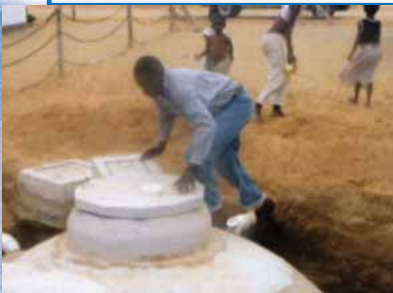
Biogas Digester installed at the Omdel settlement in Henties Bay.
